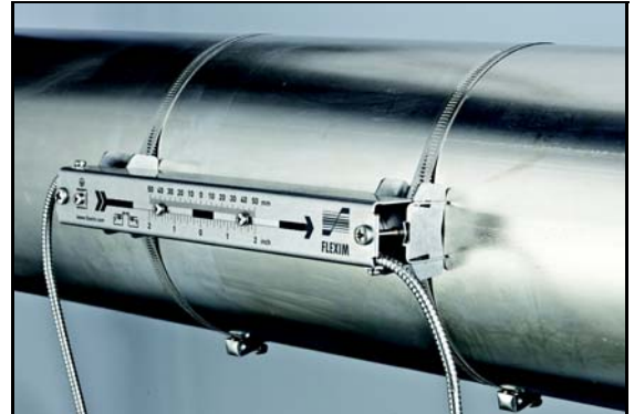
Measurement with transducers mounted by PermaRail
